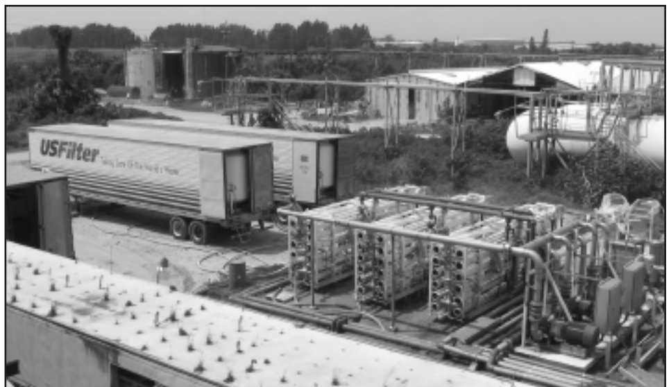
About half the Piney Point treatment system that includes media filtration, 2-pass RO, and off-site ion exchange regeneration.
