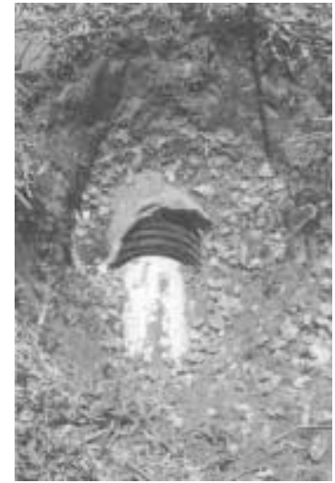
Figure 2. An illicit connection with a drainfield.
