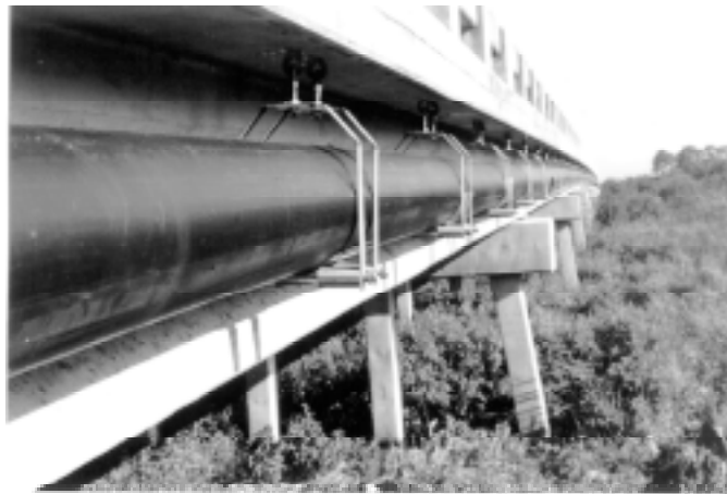
16-inch polyethelene forcemain suspended from FDOT bridge.
