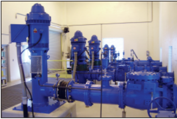
The high-service pumping facilities are designed to allow phased expansion as the plant capacity increases.
